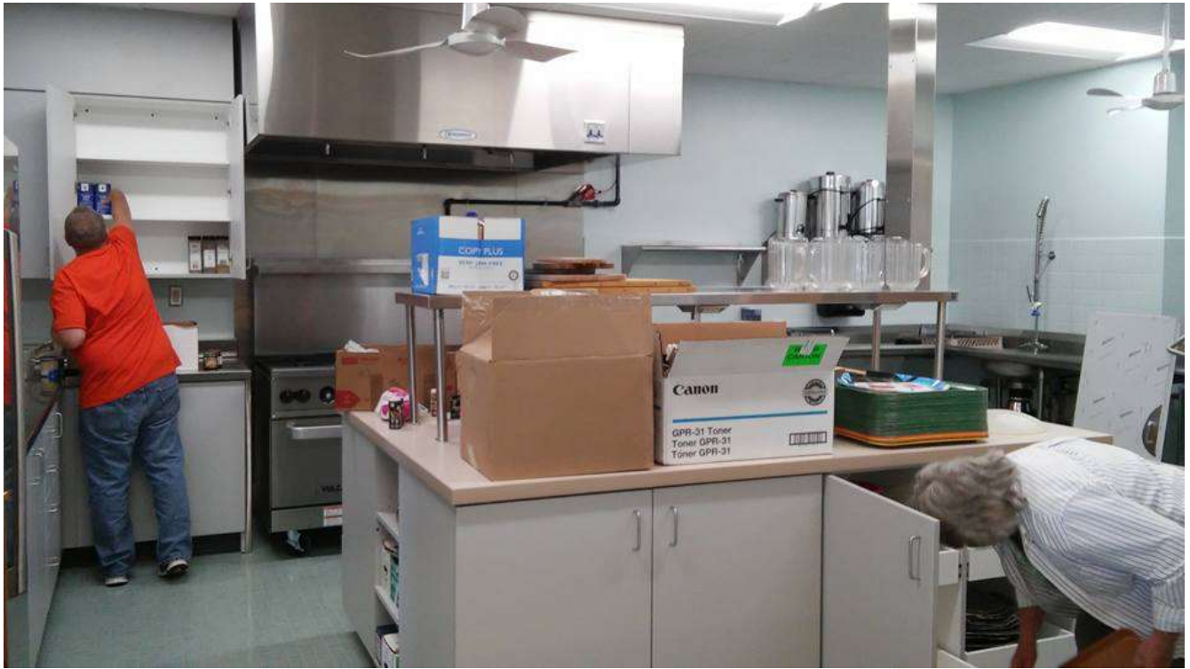
Pastor Dean and Chris Anders hard at work putting the kitchen back together, in preparation for Road Home.
